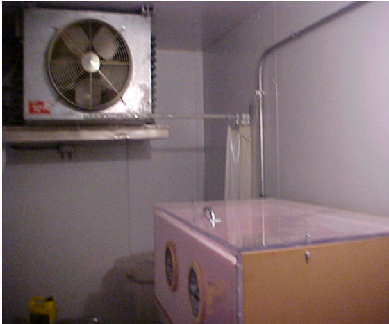
1. Temperature Regulated Box and Fan
